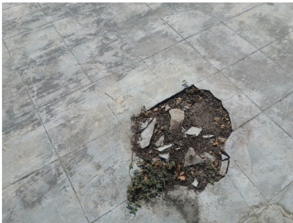
Fig 3 Delaminated Areas on the Slab
