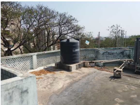
Fig 9 Water patches close to water tank
