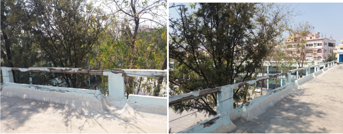
Fig 11 and 12 Corrosion of the railing of the Parapet Wall
