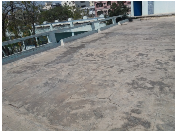
Fig 2 Cracking on the Slab Top
