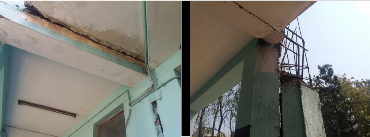
Figs 16 and 17 Expansion Joints-Leakage of Water from Roof Top/Floor above
