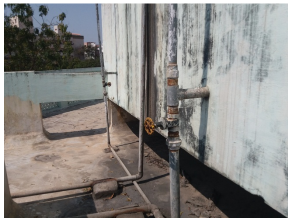
Fig 10 Corroded GI Pipes
