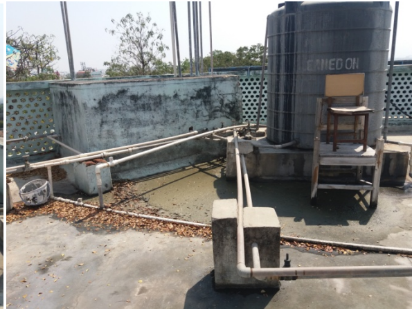
Fig 8 Overflowing of water from tank
