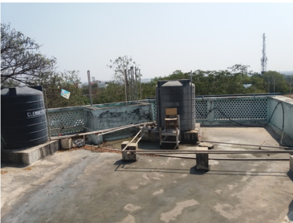
Fig 7 Water Stagnation near Water Tank
