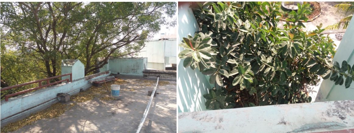
Fig 14 and 15 Invasion of Trees on the Building
