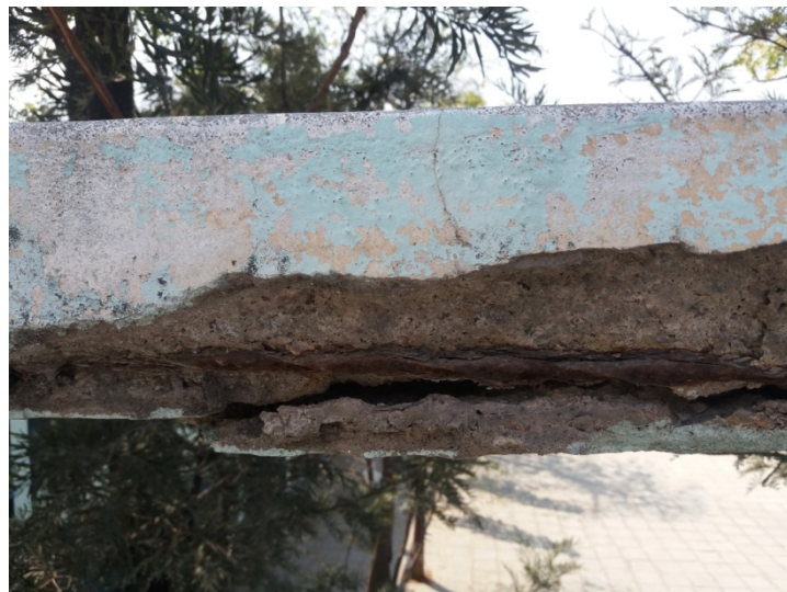
Fig 13 Loss of Diameter of Reinforcement-Severe Corrosion
