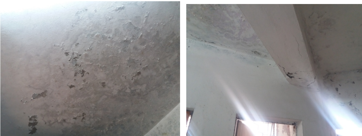
Figs 18 and 19 Dampness in the Slab due to septic water from the Toilets in First Floor
