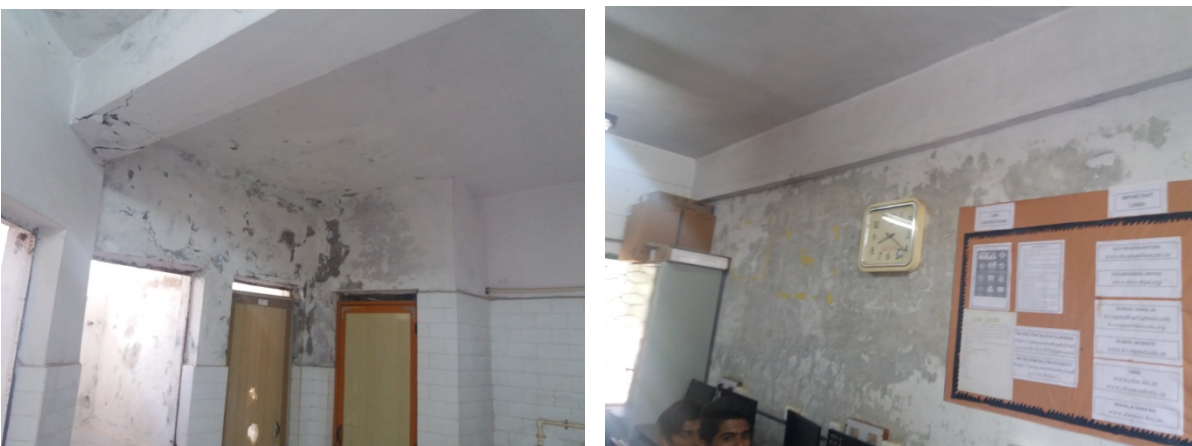
Figs 20 and 21 Dampness in the Walls
